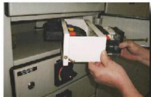
3 pole Plug-In / Demountable Type Circuit Breaker Feeder.
